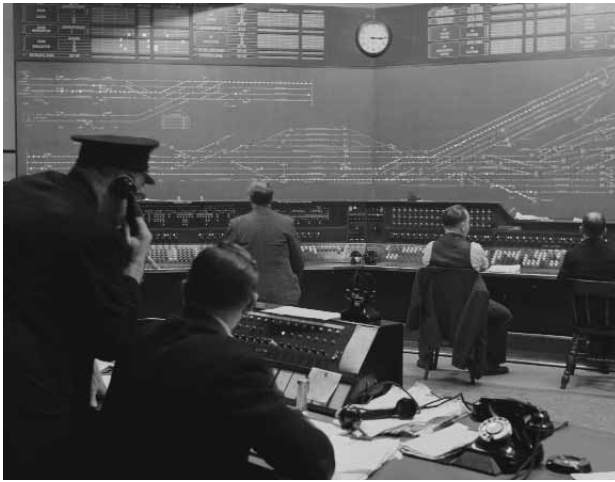
Modern signal control room at York station, 1951.
